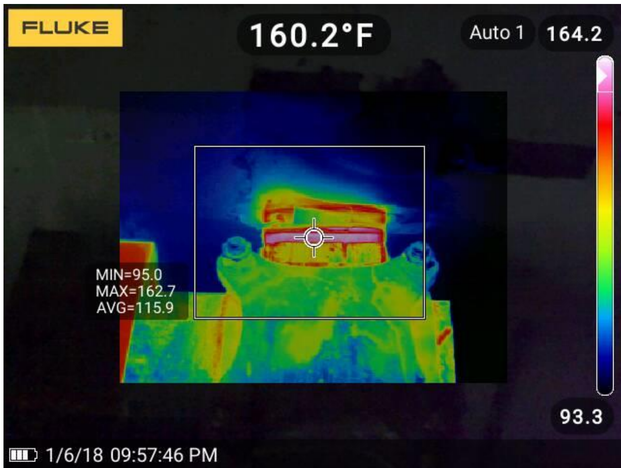
Figure 5-13 Thermal image of the bus bar from the view of the tunnel
