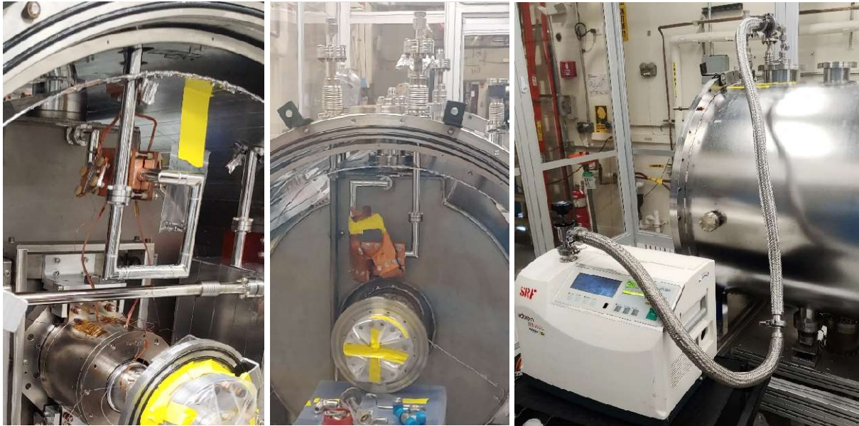
Figure 74. Internal cryostat helium system plumbing connection process: solenoid intercept loop (left), cathode bellows intercept loop and fast cooldown line and respective top connections (center), helium leak checking conflat joints (right).
