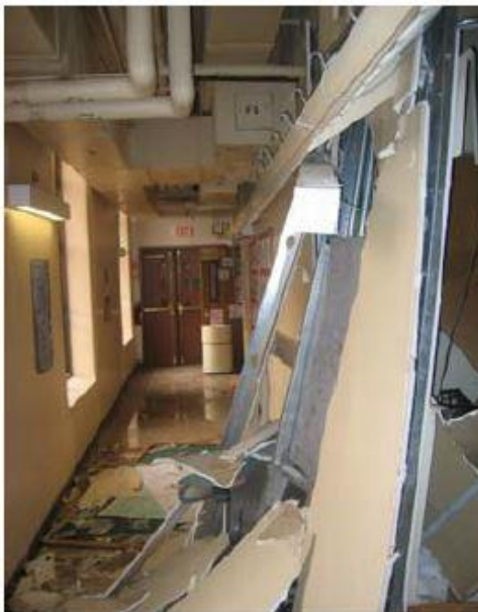
Figure 2 - Hallway Outside Laboratory Showing Explosion Damage
