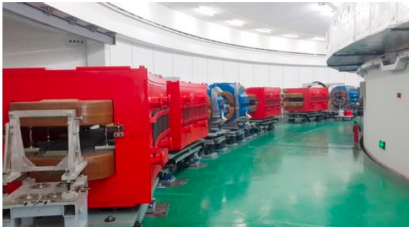
Figure 10: The dipoles and quadrupoles installed in the tunnel.
